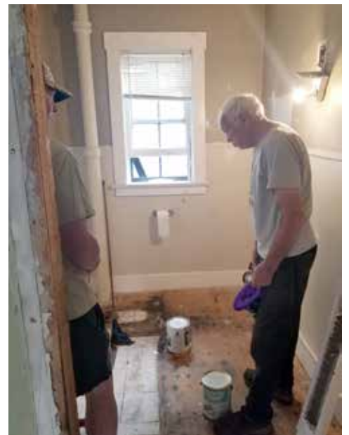
Bill Snowdon hard at work on the bathroom renovation in the Boultenhouse Heritage Centre apartment.
